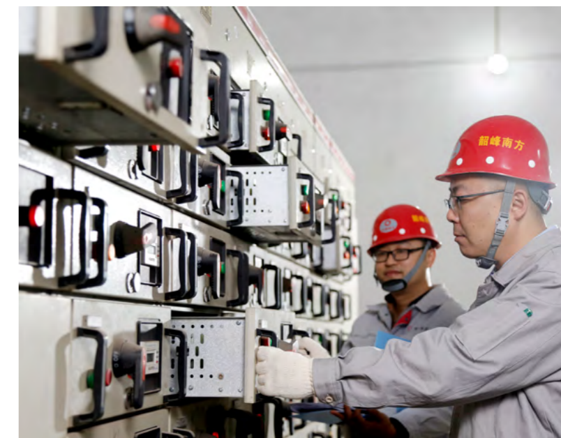
© Hunan Shaofeng South Cement Company Limited employees are checking the equipment in the electrical room
